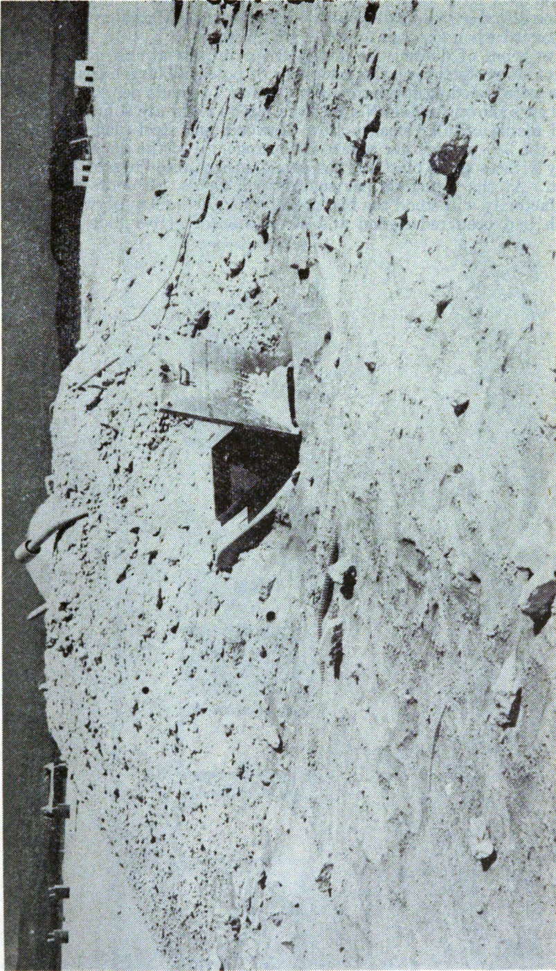
SLIDE No. 24.—Damage to structure.
